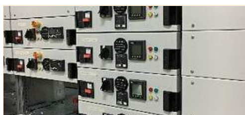
H.VIR® implanted on LV switchboards.
