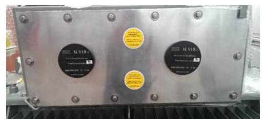
H.VIR 85® on oil transformer.
