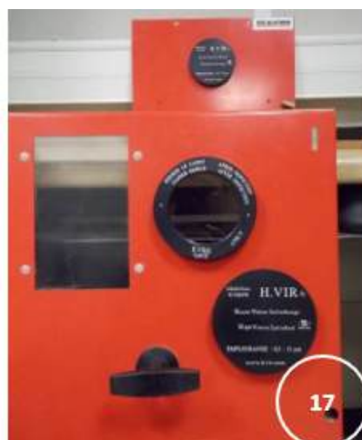
Electrical equipment ready for inspection.
